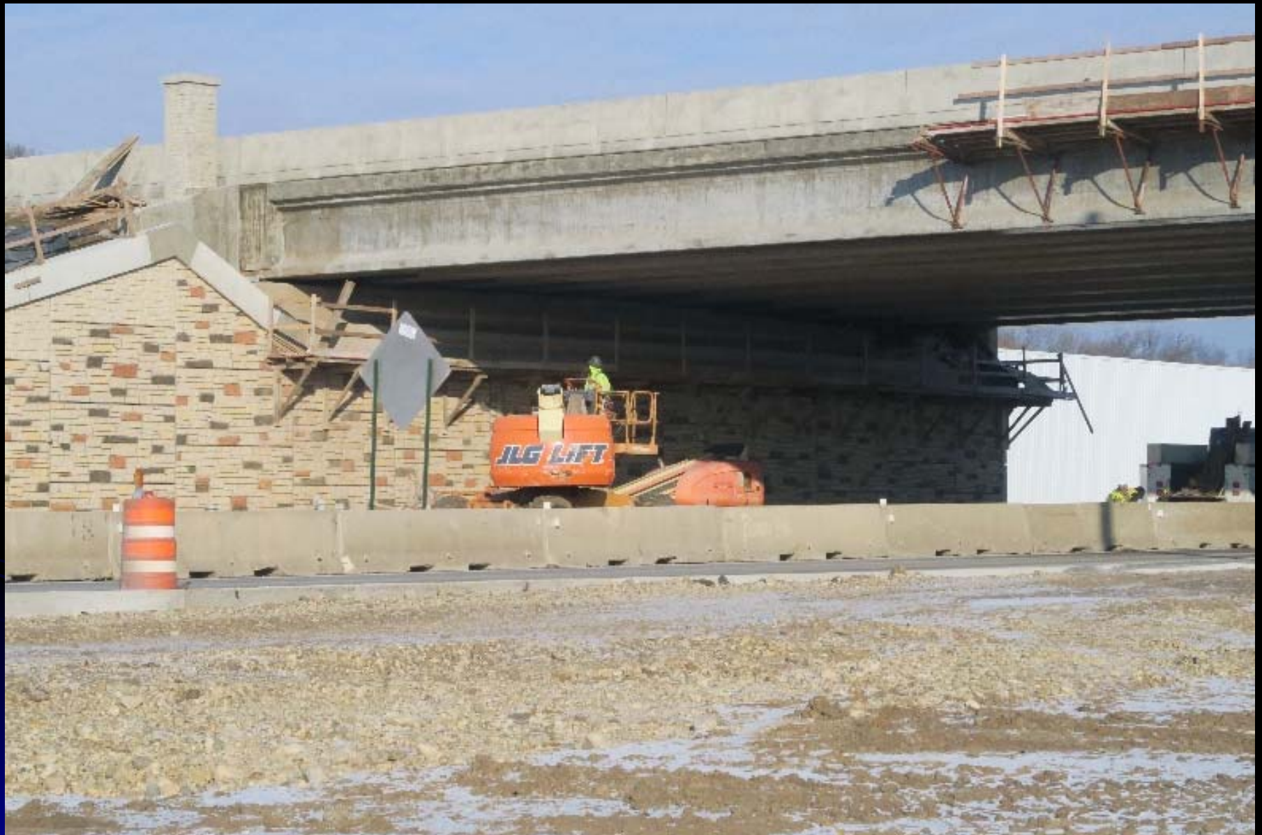
Crews install bridge drainage pipes under the new IL 31 bridge between warm and cold weather on LMP Section B-2
